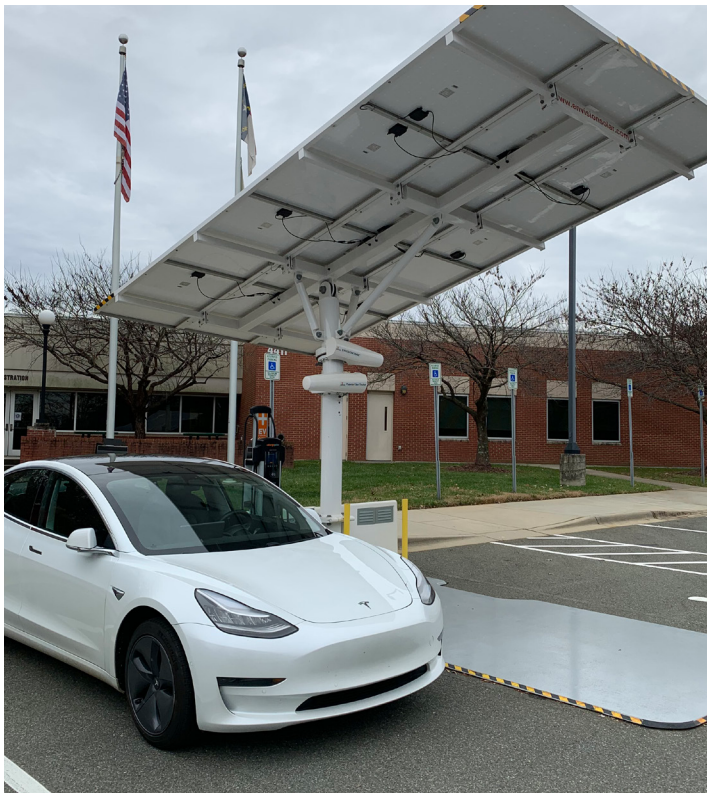
Solar-powered charging station in Charlotte, North Carolina.
