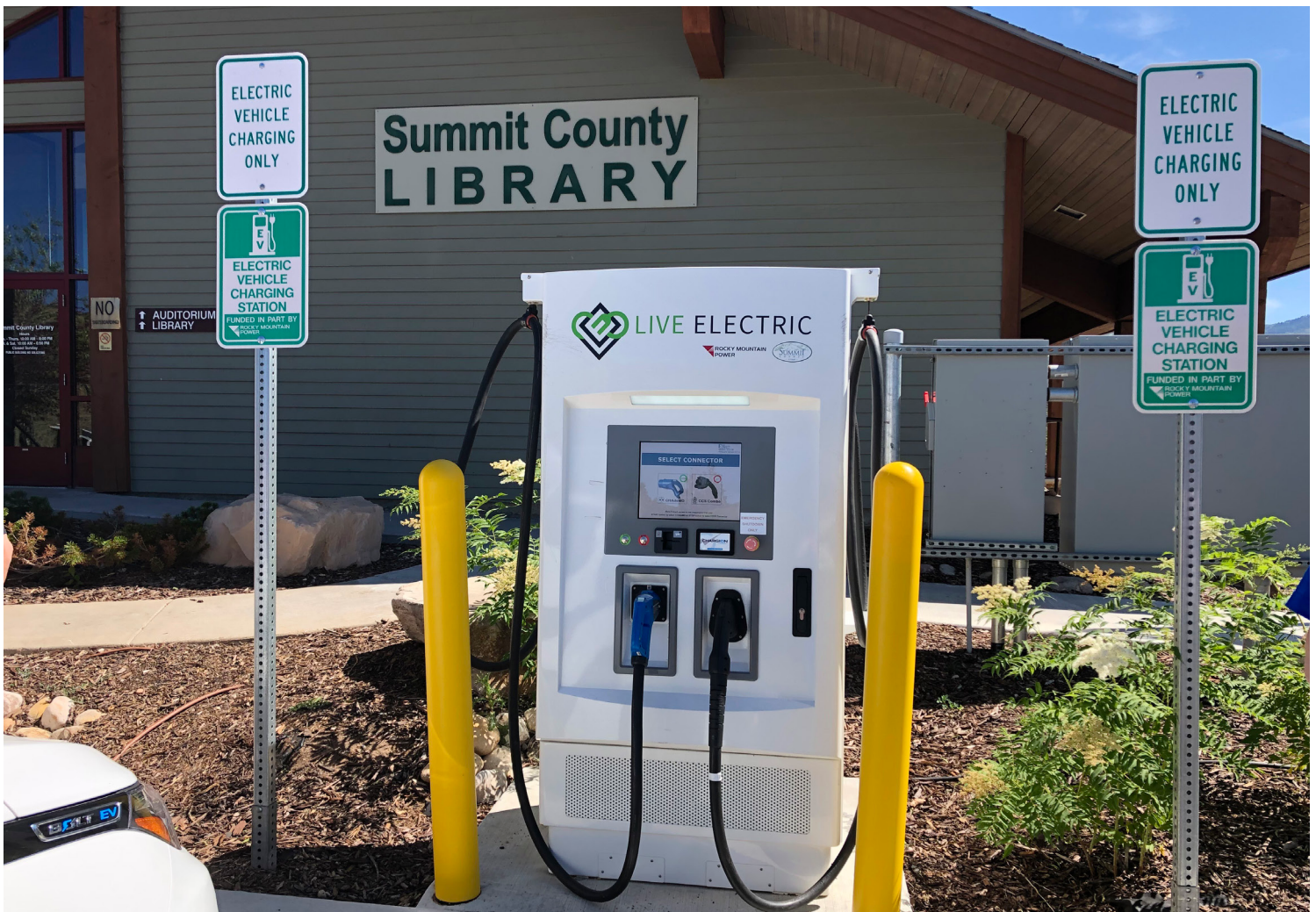
A charging station at a library in Frisco, Colorado.
